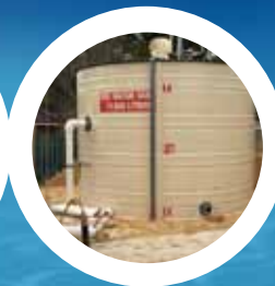
Level Indicator - Signage Ventilation - Pipe Supports
